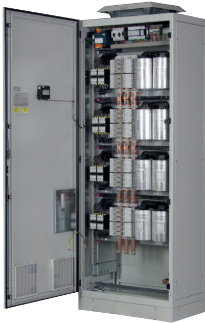
Batteries de compensation
